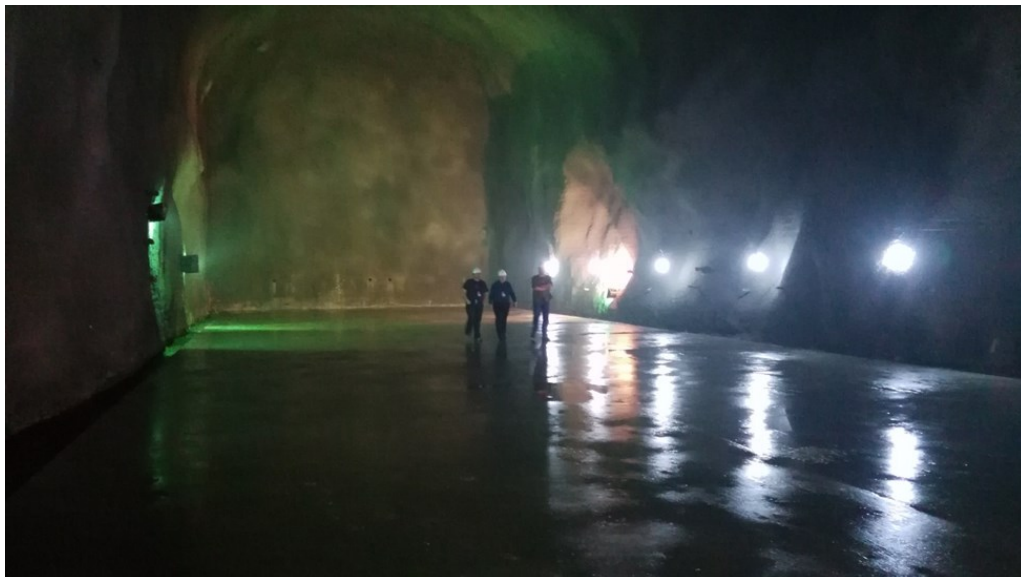
Dan Robertson, Michael Wiescher from JINA-CEE and Frank Strieder from the South Dakota School of Mines & Technology in the 14x14x130m excavation that will house the JUNA accelerator facility.
